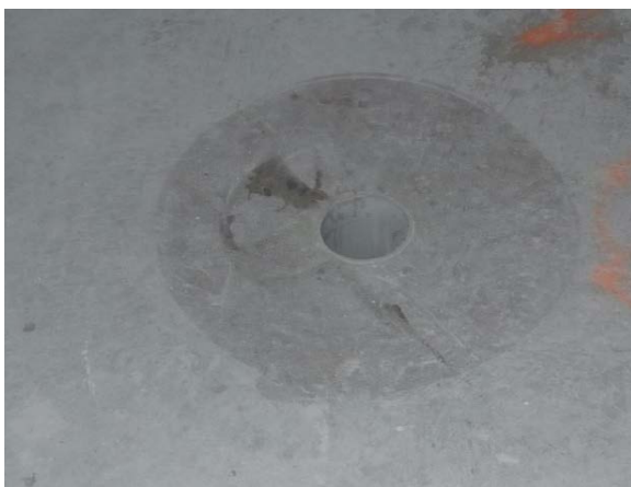
Figure 2 Example of a missing drainage flange
