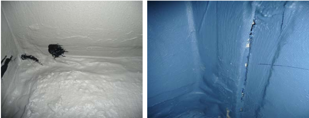
Figure 1 Examples of poorly prepared substrates
