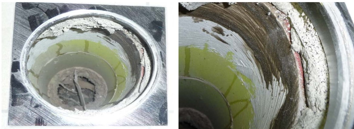
Figure 3 Incorrectly installed membrane at drainage flange
