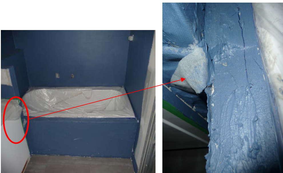
Figure 5 Example of poor workmanship around a bath
