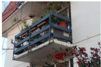
Replace Rotten Handrails to Balconies
