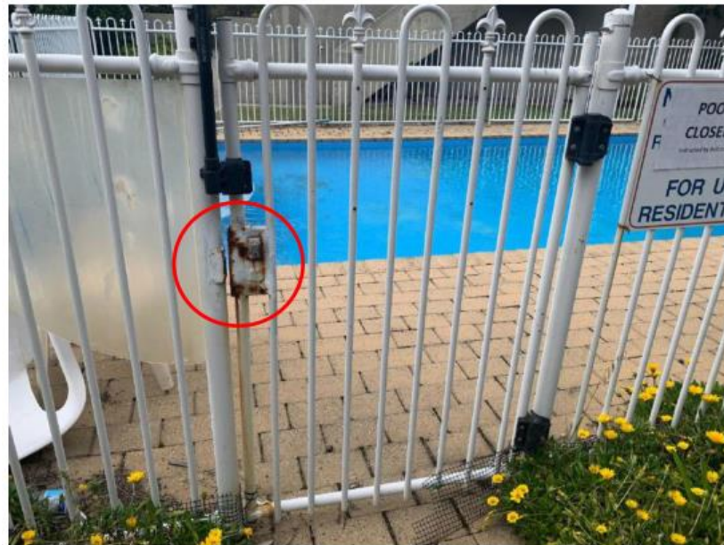
Photo 22 - rectify pool gate lock corrosion
