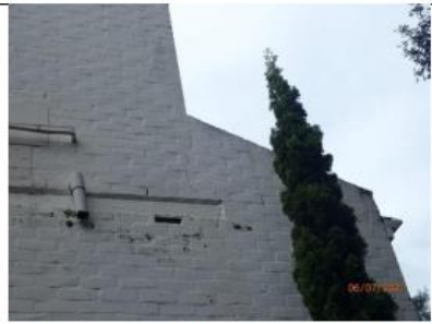
Assess Rectification of Damp to Walls
