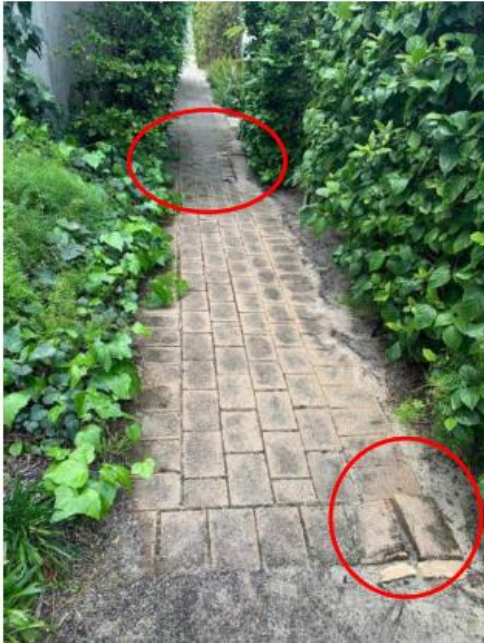
Photo 9 - rectify 3m2 of pavers to path north of Unit 8
