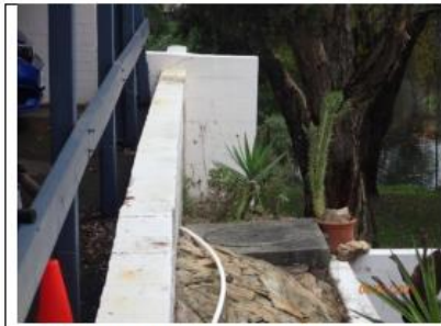
Investigate Movement in Retaining Walls
