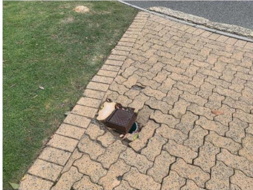
Photo 18 - rectify pavers in entry drive near Unit 17
