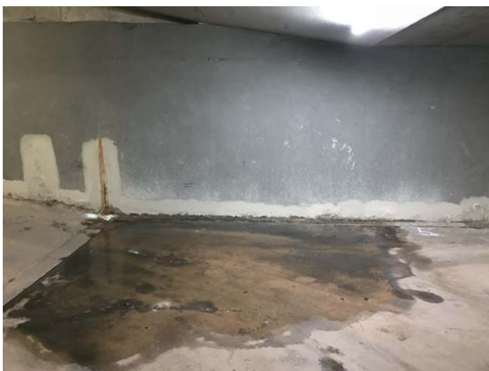
Water seeping through the basement wall
